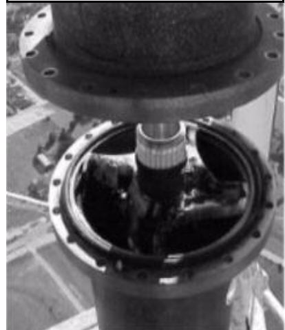
KTVT (Cedar Hill ) burnt coax for high definition TV antenna after initial transmitting test.
